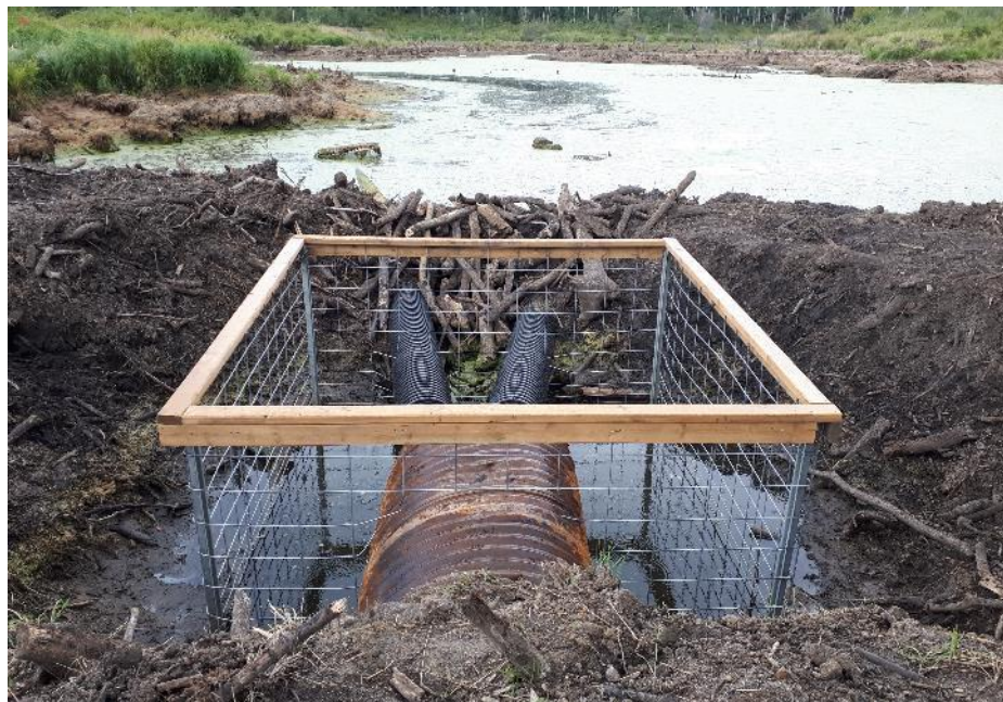
Figure 13: Double pipe combination device for higher capacity (Location: Cooking Lake Blackfoot Provincial Recreation Area, Alberta)
