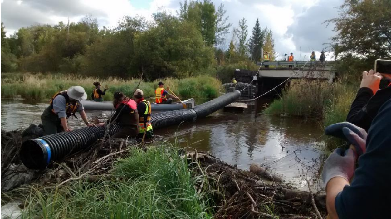
Figure 3: Constructed pond leveller being placed into the dam and wetland. The wire cage (intake end) will be lowered and secured with weights to be kept at the bottom of the pond. The outlet end will be secured in the dam (Location: Lac Ste. Anne County, Alberta).
