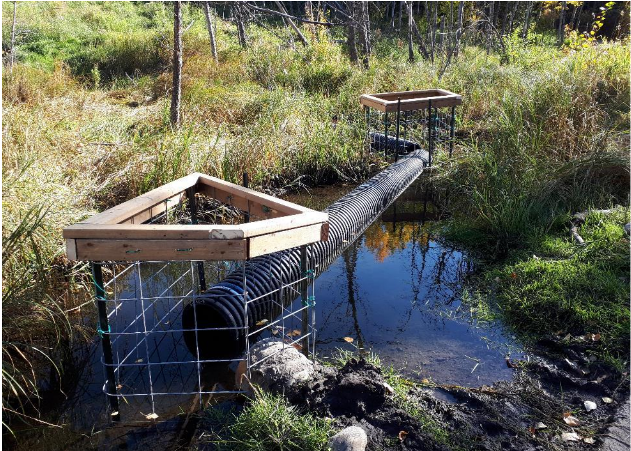
Figure 6: Multi-intake combination device (Location: Calgary, Alberta).
