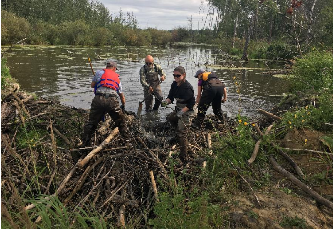
Figure 1: Practitioners creating a notch in a beaver dam prior to installing a pond leveller (Location: Parkland County, Alberta)
