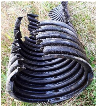
Figure 8: Single wall pipe, chewed through by beavers
