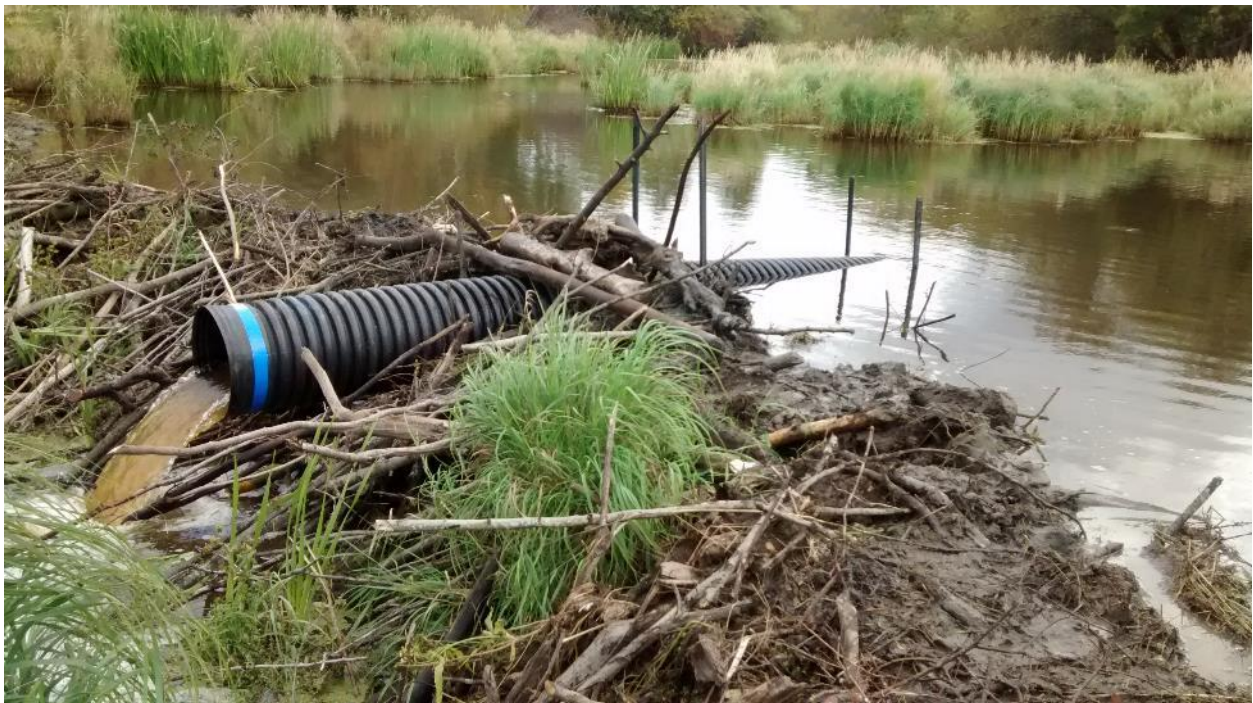
Figure 4: View of the outlet end of the pond leveller after being secured in the dam (Location: Lac Ste. Anne County, Alberta).
