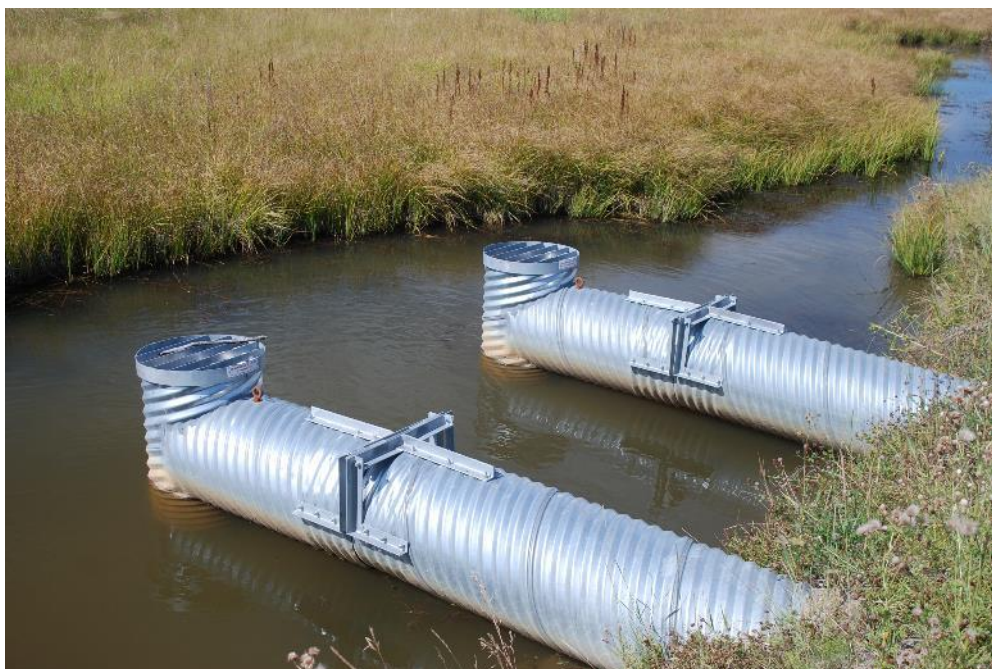
Figure 11: Beaver-Proof Culvert Add-on installed while doing a routine replacement of old culverts at this road crossing. The road had been experiencing flooding resulting from beaver plugged culverts. The installation happened in 2012 and cost $35,000 and has not required any further maintenance. Installed costs recouped, now saving the county $5,000-10,000 annually (Location: Foothills County, Alberta) 17 .
